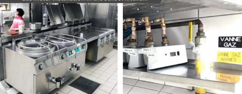
Gas meter installation in the school kitchen.
