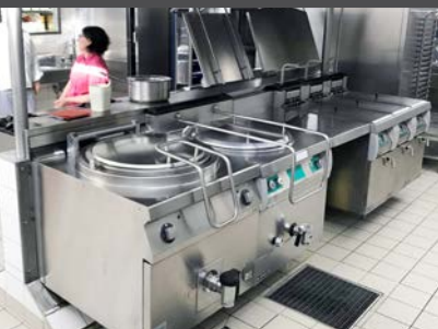
Gas meter installation in the school kitchen.
